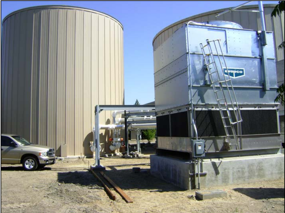
New Cooling Tower and TES Tank #2
