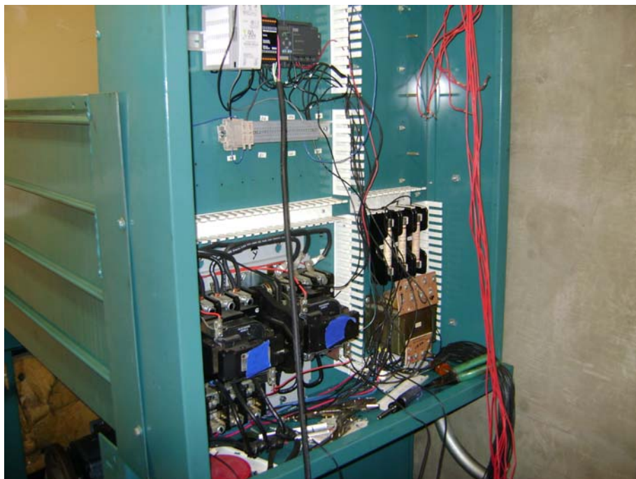
Atherton– Updated Electrical Motor Panel for Lift
