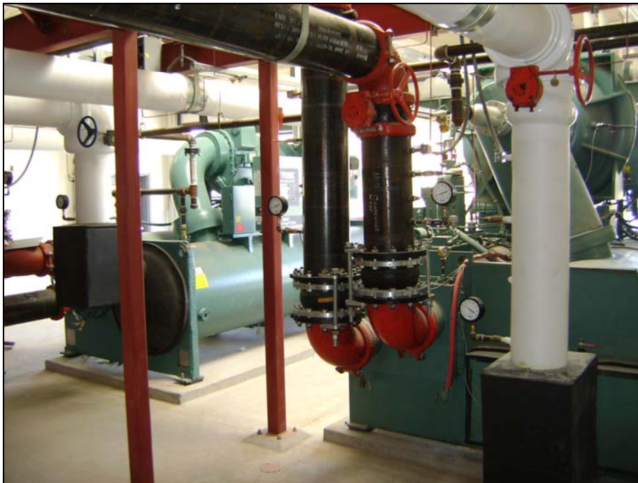
Chiller Room Interior
