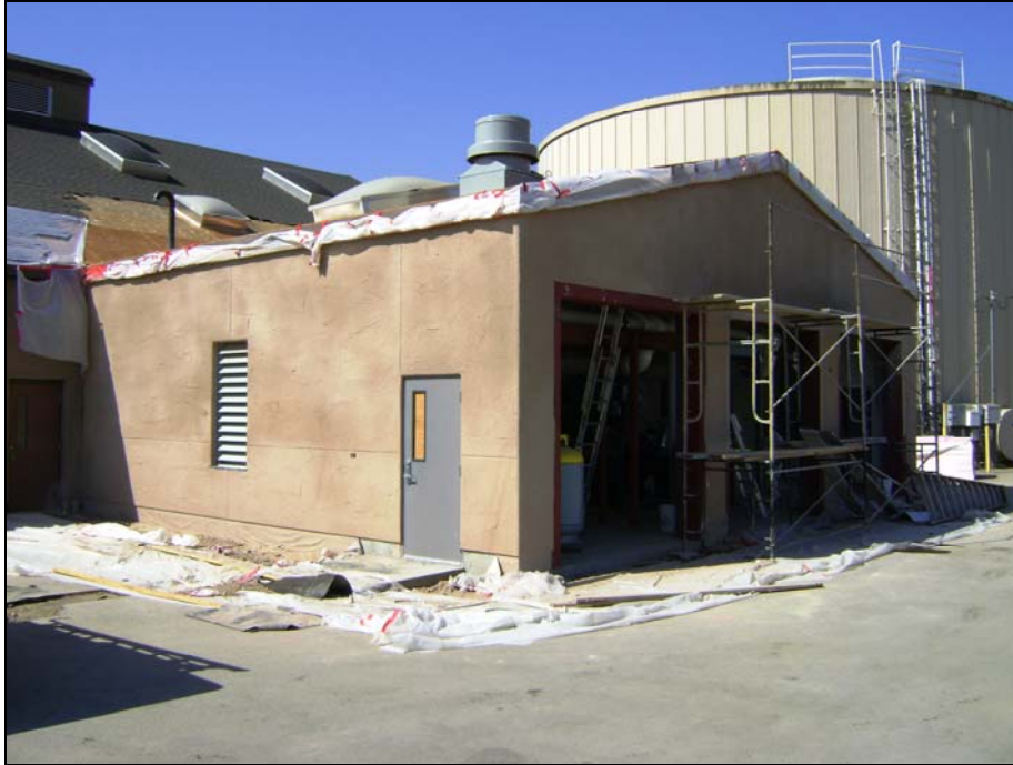
Chiller Building Addition
