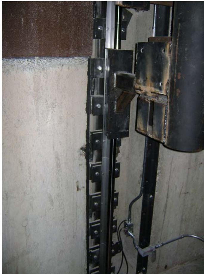
Atherton– View of New Guide Rail Inside Pit Lift
