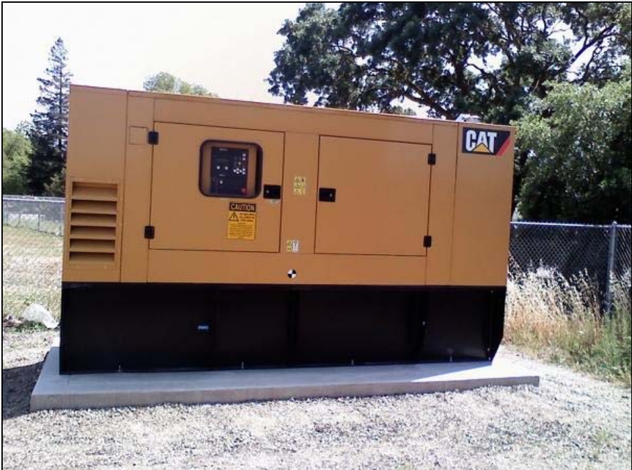
New Generator Installed
