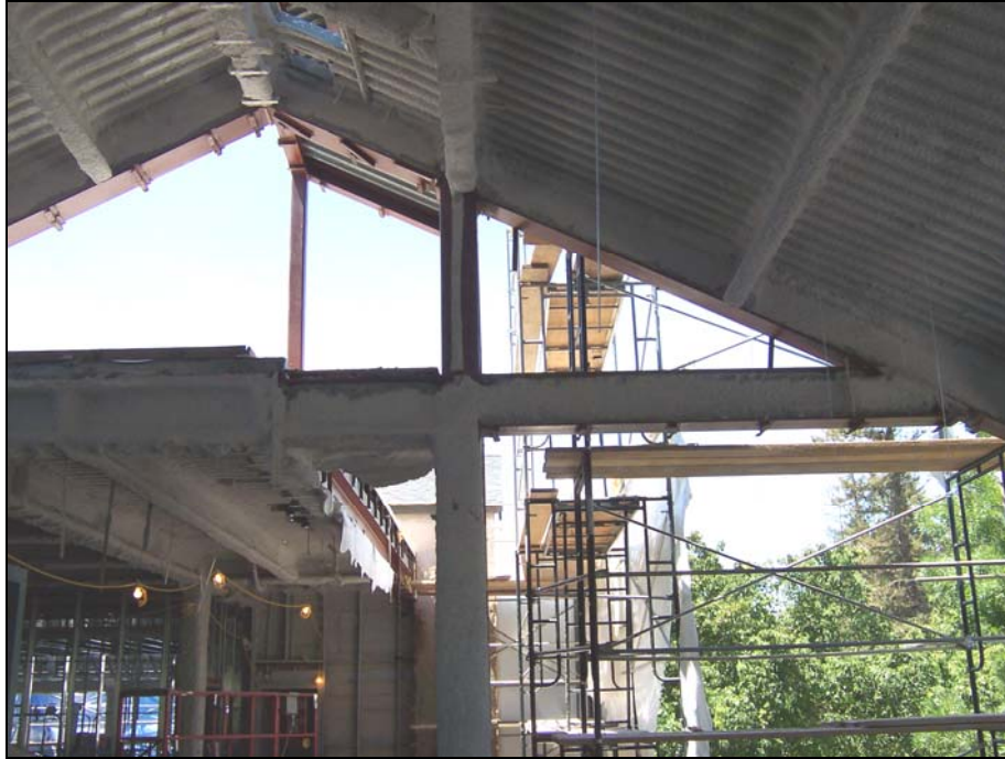
Rusted Studs Were Removed at Exterior Walls
