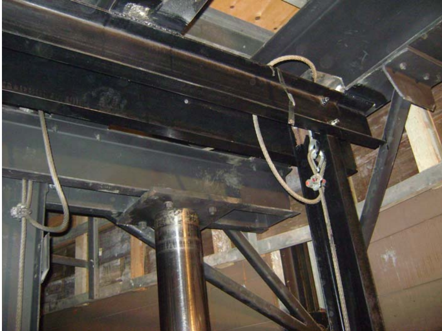
Tillie Lewis – Bottom View of Lift Inside Pit Lift
