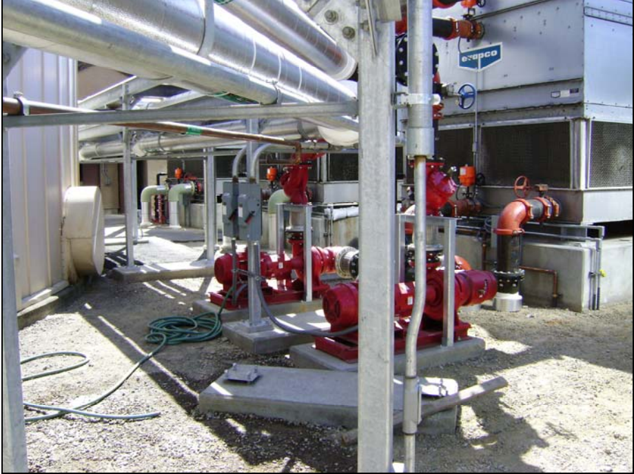
Mechanical Yard Piping and Pumps
