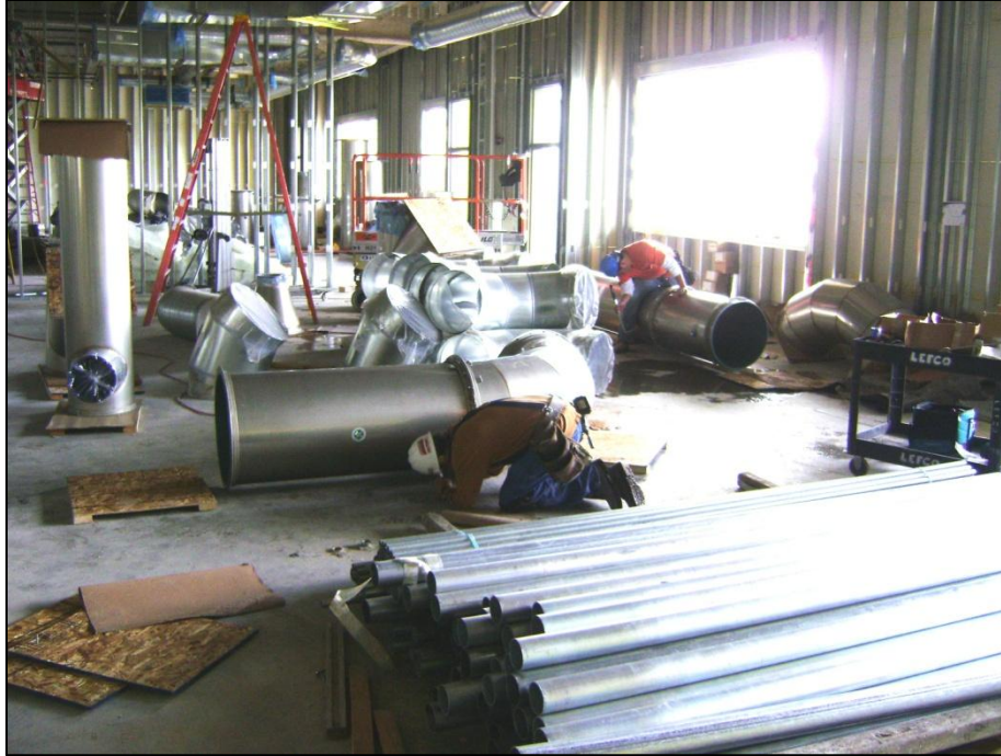
Stainless Steel HVAC Duct Assembly
