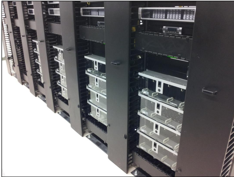
Data Center – New Fiber Optic Cable Enclosures
