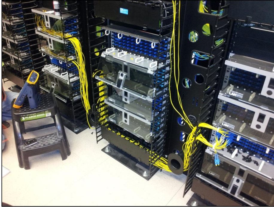
Temporary Jumper Cables Installed
