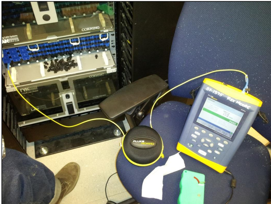
Verification of New Cable Connections
