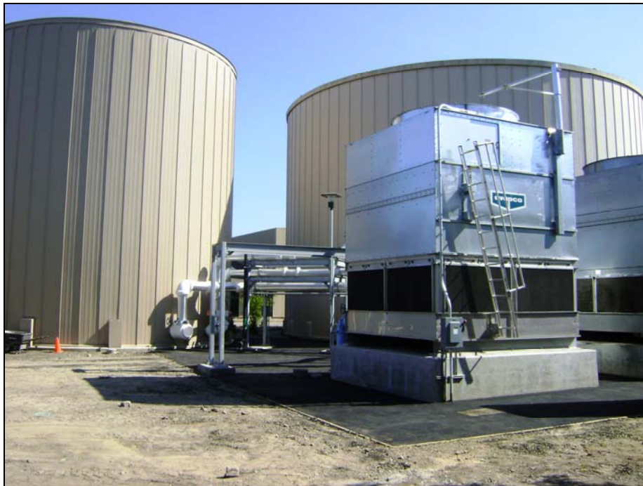
New Cooling Tower and TES Tank #2
