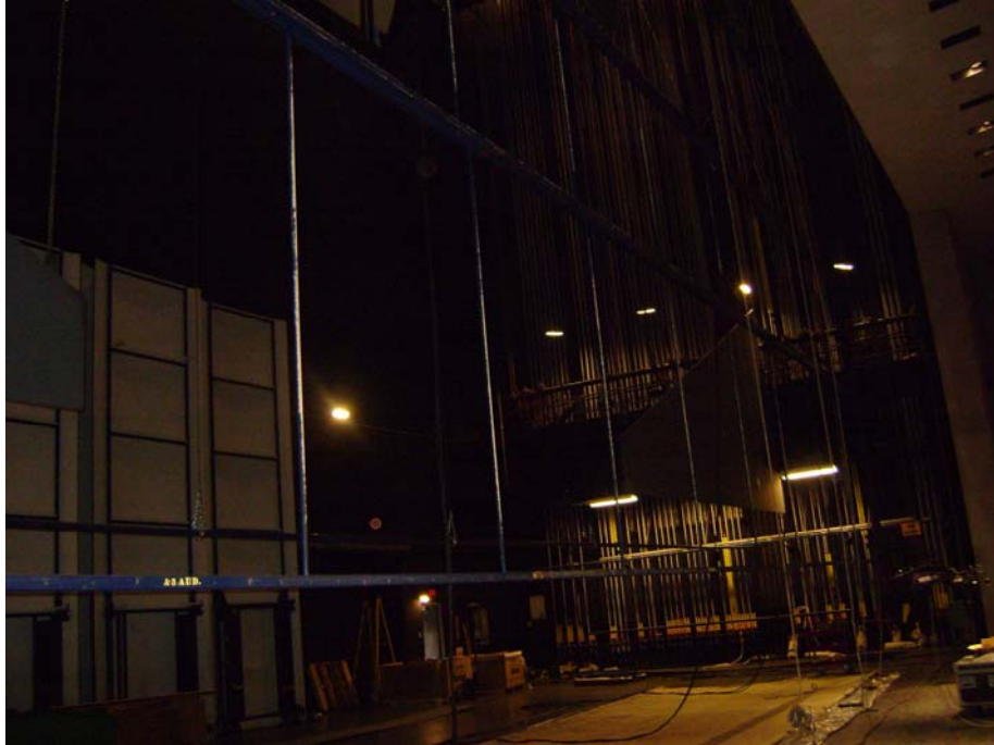
Atherton – View of Fire Curtain Frame and Rigging
