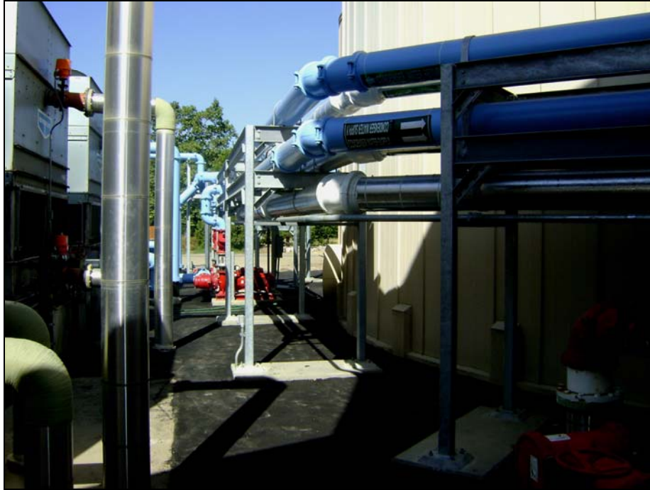
Mechanical Yard Piping and Pumps
