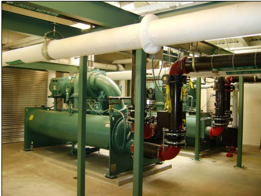
Chiller Room Interior
