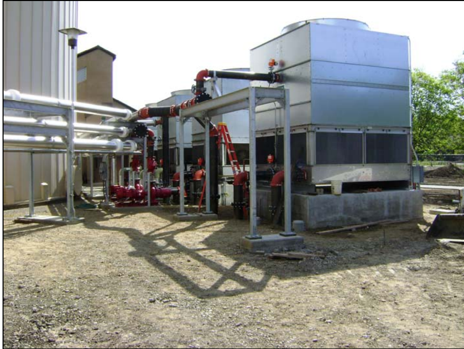
New Cooling Tower and Associated Piping
