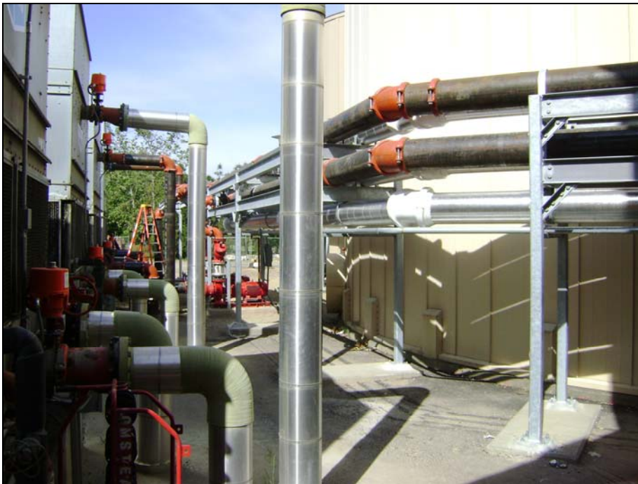
Mechanical Yard Piping
