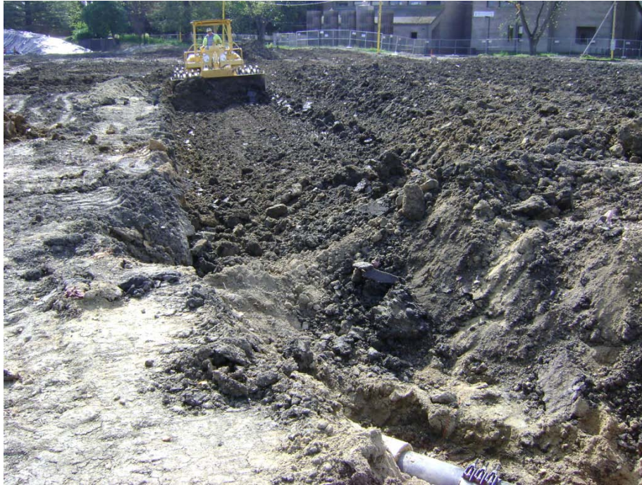
Compaction and grading of excavated building pad located at Building Wing A.
