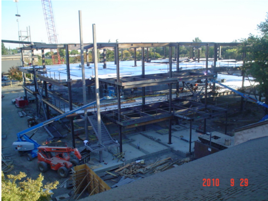
Building Wing A Structural Steel Erection for Floors One, Two, and Three
