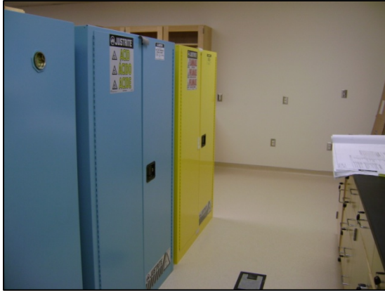
Portable 403 rear, chemical storage cabinets
