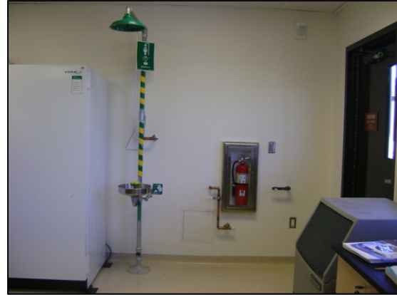
Portable 403 front, emergency shower
